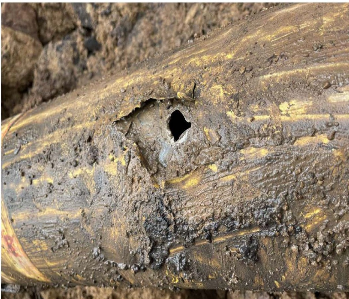
Photo 1. May 2023 Pipeline Hole
